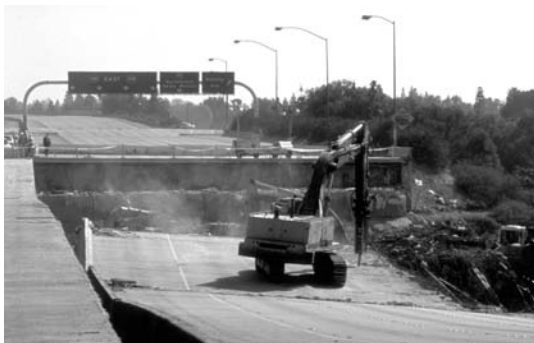
Northridge Earthquake, CA, January 17, 1994 Many roads, including bridges and elevated highways were damaged by the 6.7 magnitude earthquake. Approximately 114,000 residential and commercial structures were damaged and 72 deaths were attributed to the earthquake. Damage costs were estimated at $25 billion. FEMA News Photo
