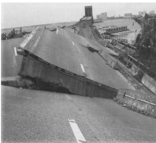
Biloxi, Mississippi, USA. On Aug 30, 2005, the Louisiana and Mississippi coasts were hit by a category 4 storm with maximum winds at 140 mph. This bridge was no match for Hurricane Katrina. This vital link connecting Biloxi to Pascagoula was swept 30 feet off its pylons and cast into the sea. The bridge remains closed eight months after the storm.
