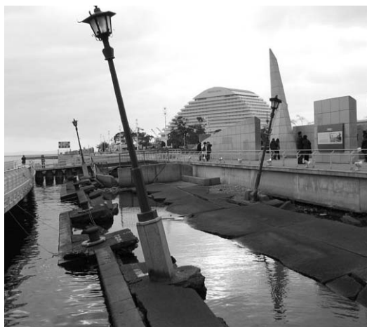
Kobe Earthquake Memorial Park, Japan. On Jan 17, 1995, the city of Kobe was struck by a magnitude 7.2 earthquake. The memorial is an area of the Meriken Pier which was hit and has been preserved in its damaged state. It relays the tragedy of the disaster and the city's subsequent restoration. Although the destruction to the port of Kobe was devastating, the entire city was rebuilt in just 2 years!
