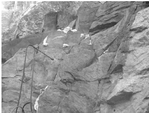
Figure 2. Staged PUR pumping underway. The two-part resin mixes at the delivery tube, and permeates the rock mass.
