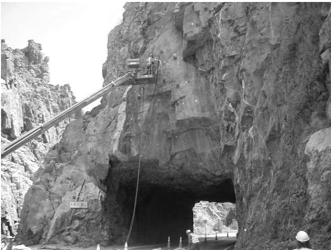
PUR injection in the highly jointed rock mass above the Poudre Canyon Tunnel west of Ft. Collins. The left tunnel abutment and the rock mass extending approximately 20 feet above the portal were treated.
