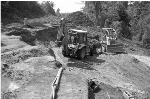
Super nails and micropiles cantilever a GRS wall over a slide scarp.
